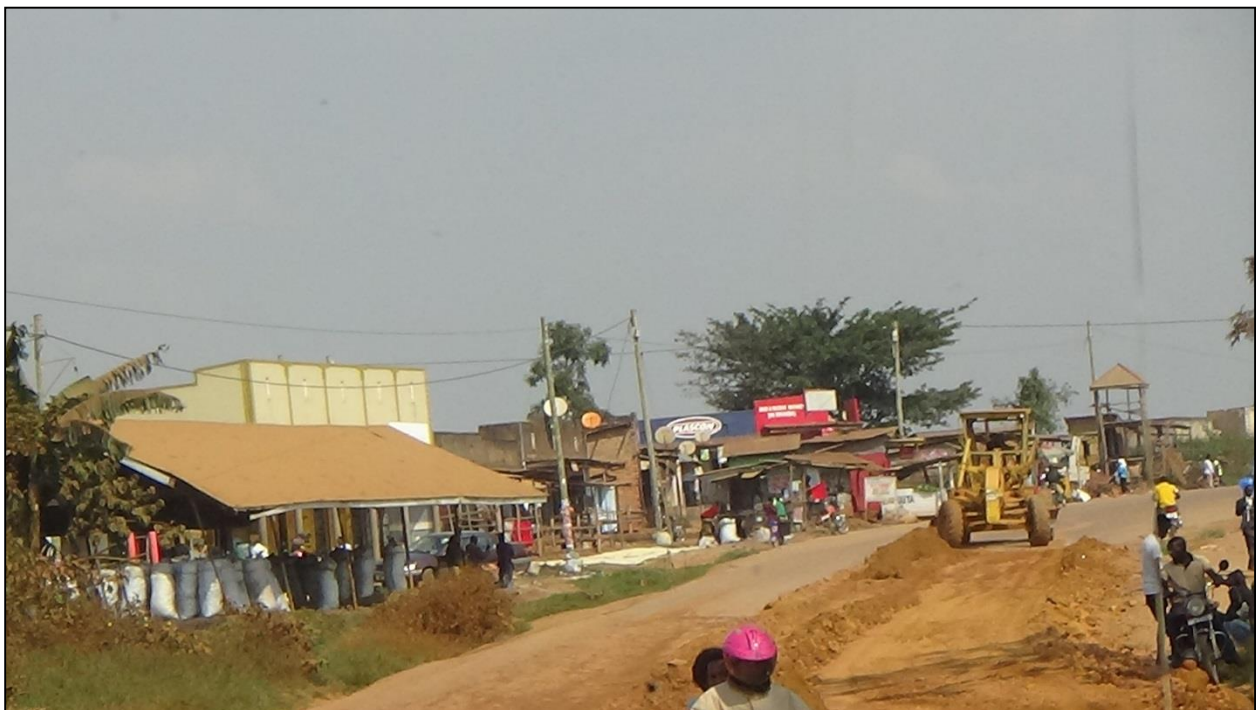
Figure 2: above shows on-going maintenance of the carriage way to improvement on its motorable condition for public traffic.
