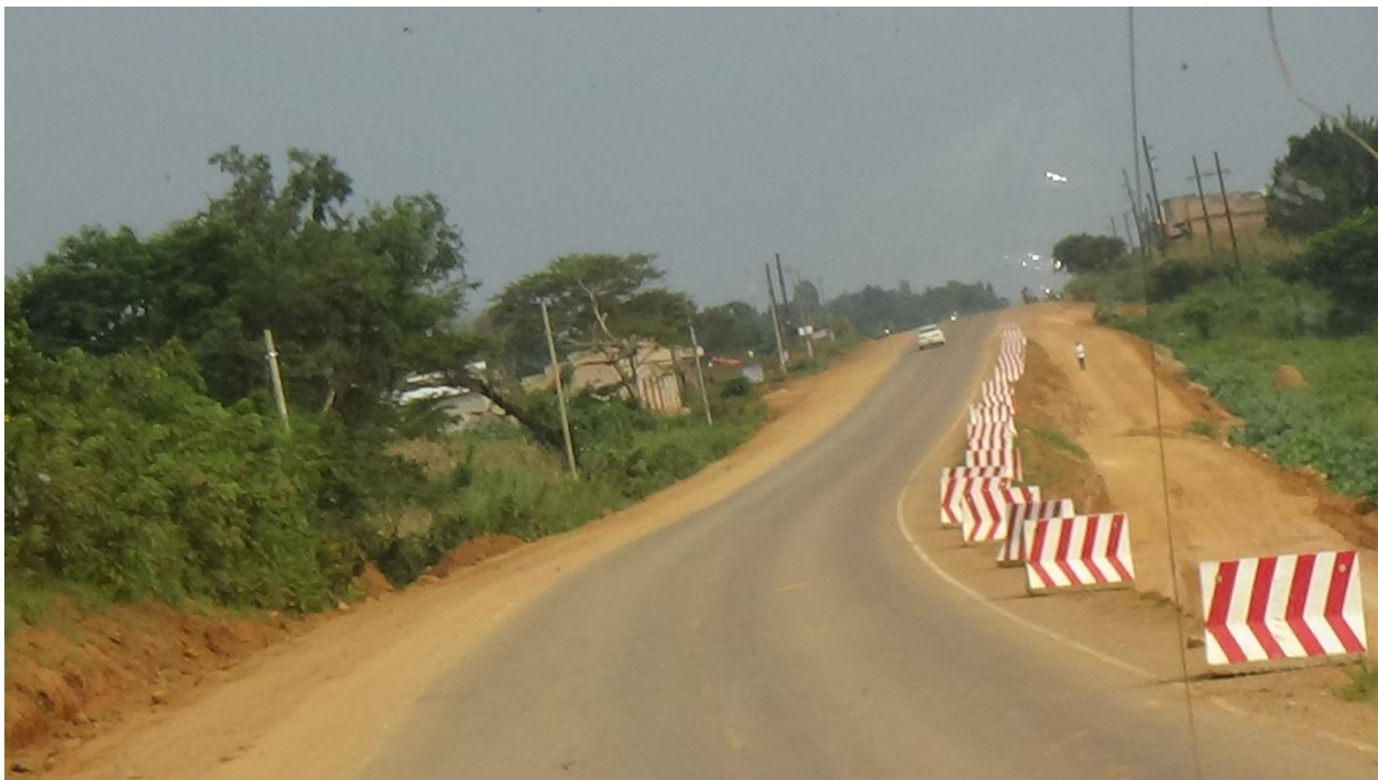
Figure 4: above showing new-jersey barriers provided to segregate moving traffic from the work section along the project road.
